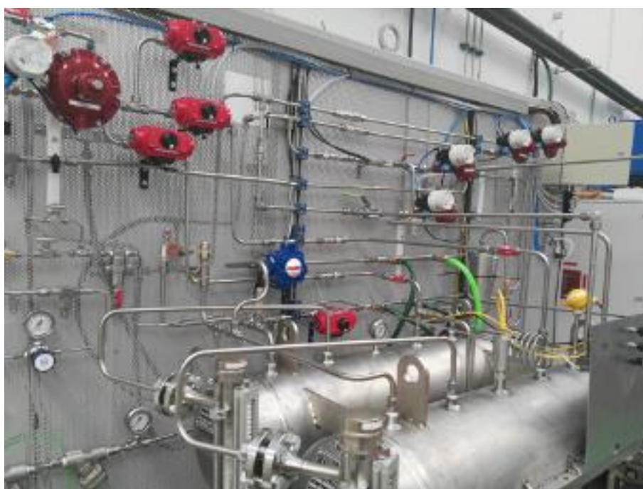
Figure 2. Pilot test bench, intermediate scale, erected at FHA facilities
