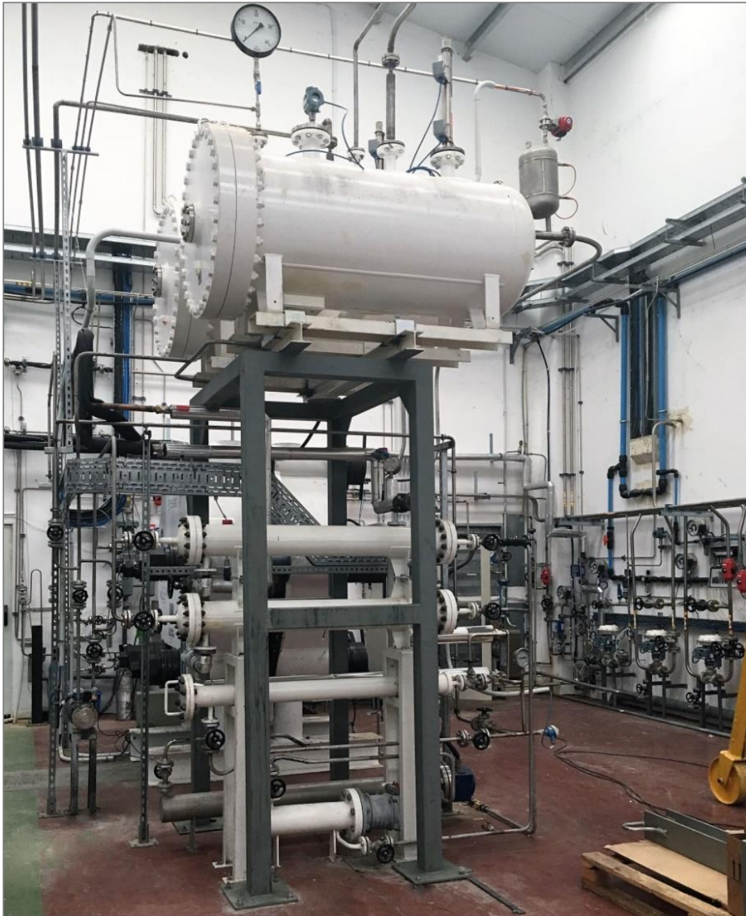
Figure 2. Test bench (FHA facilities)
